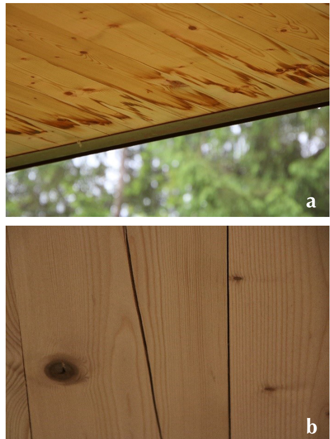
Figure 4. (a) Damage caused by exposure to moisture into the end grain of the CLT panels near the bottom of the overhangs; (b) splits in the surfaces of the CLT panels caused by changes in equilibrium moisture content inside the building.
