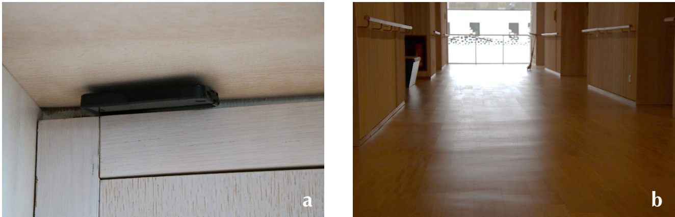
Figure 3. (a) A gap between a door and the ceiling; (b) ceiling and floor showing waving in the fifth floor due to the impact of accumulated shrinkage and swelling of CLT boxes.
