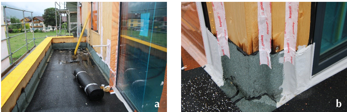
Figure 7. (a) Flashing used in balconies; (b) visible damage caused by water exposure in balconies.
