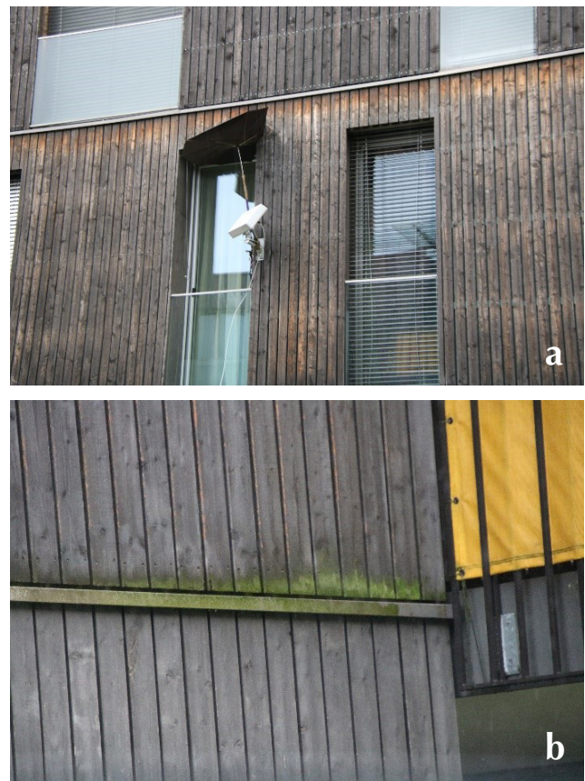
Figure 1. Direct exposure to sunlight and moisture accumulation on siding leading to (a) discoloration and (b) blue, black, or green staining.
